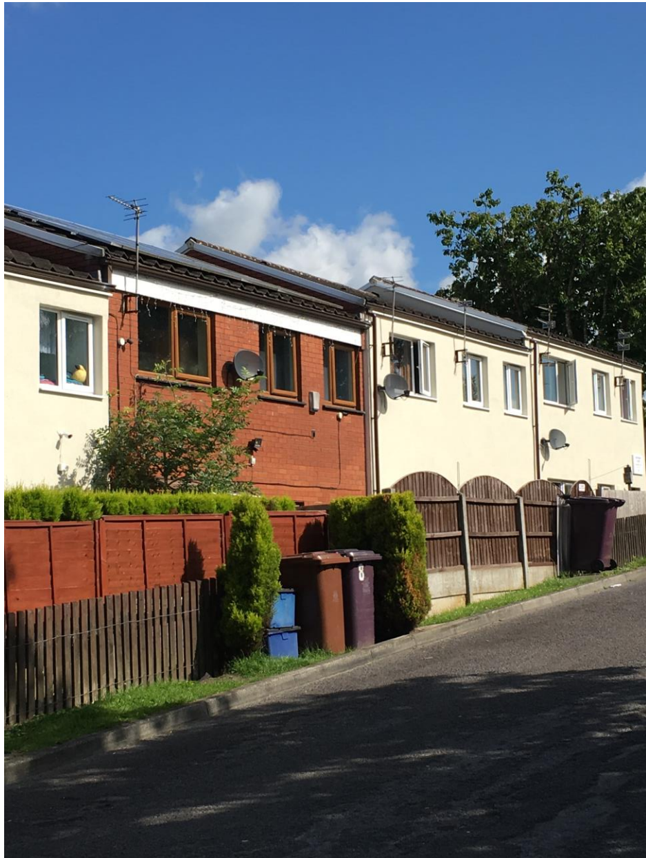
Figure 1. Result of renovation works at Padiham, showing the difference between a privately owned, non-renovated house, (brick structure), and the renovated ones with external insulation.
